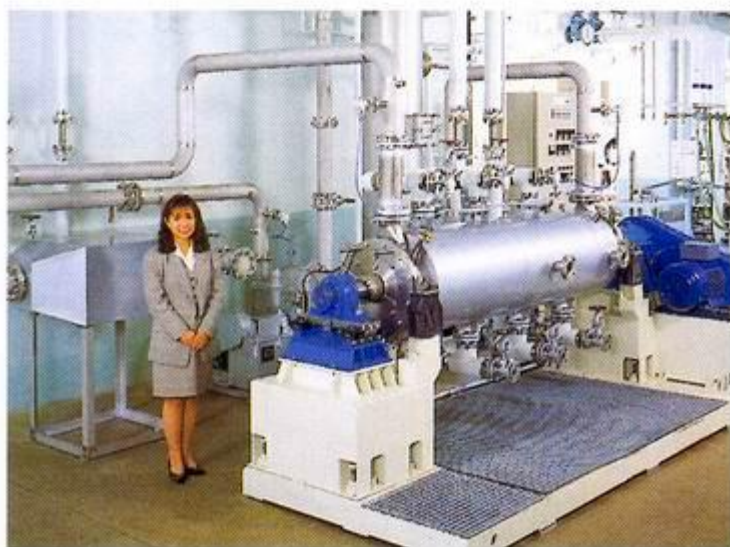
Fig. 1 - Flash Drier mod. FD 4/20, general view
